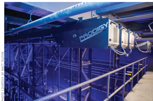
ETC Prodigy Hoists installed at Phillips Exeter Academy's Goel Center for Theater and Dance.
