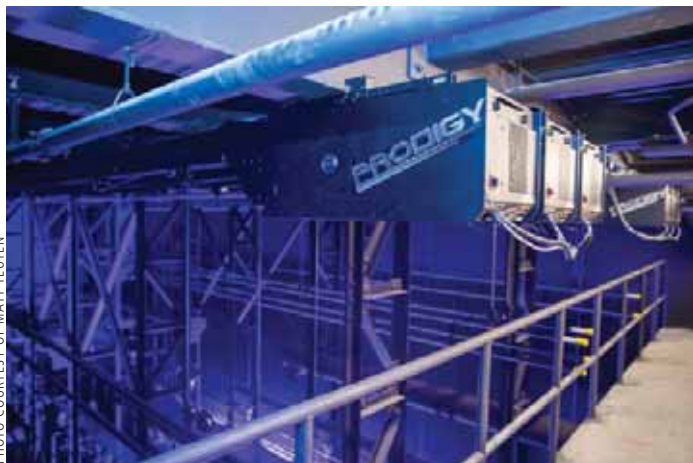
ETC Prodigy Hoists installed at Phillips Exeter Academy's Goel Center for Theater and Dance.
